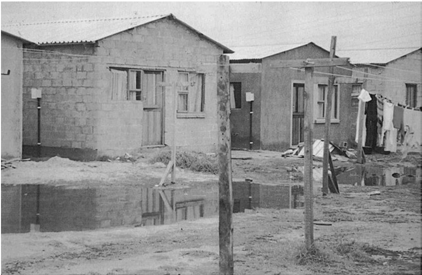
Figure 5.1 Noma's house with problems visible: area above wall and below roof not filled in, missing ridge piece, bad workmanship above door and window.
